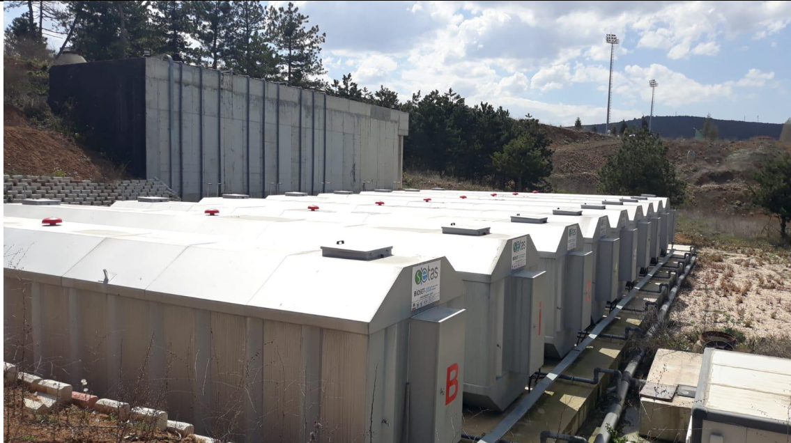
WWT Units, six packs total 900 m 3 /day Wastewater Treatment
